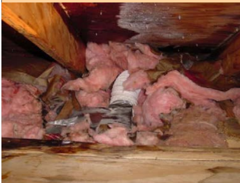
This dryer duct, venting directly into the attic space, is causing moisture issues on the roof deck and insulation. 11
