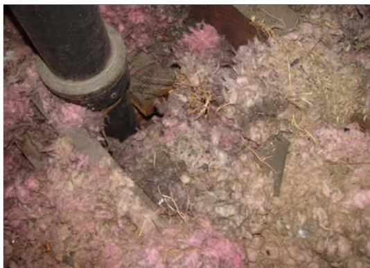
Upon closer inspection, the dirty insulation reveals an air leak at the plumbing chase. 8
