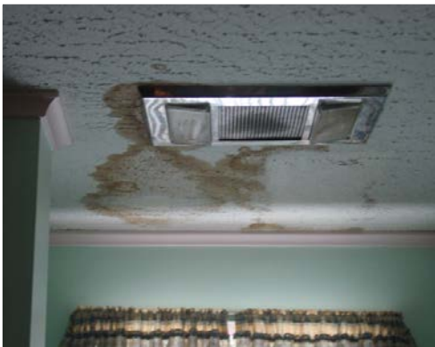
This moisture stain is an indication that the duct for this vent is not venting to the outside. 11
