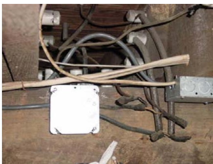
Photo shows knob and tube and other wiring hazards.
