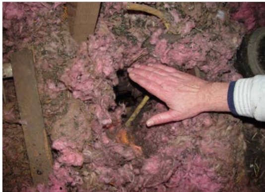
Dirty insulation revealed a gap of many square inches. With a hole this size, the attic is open to the home below. 8
